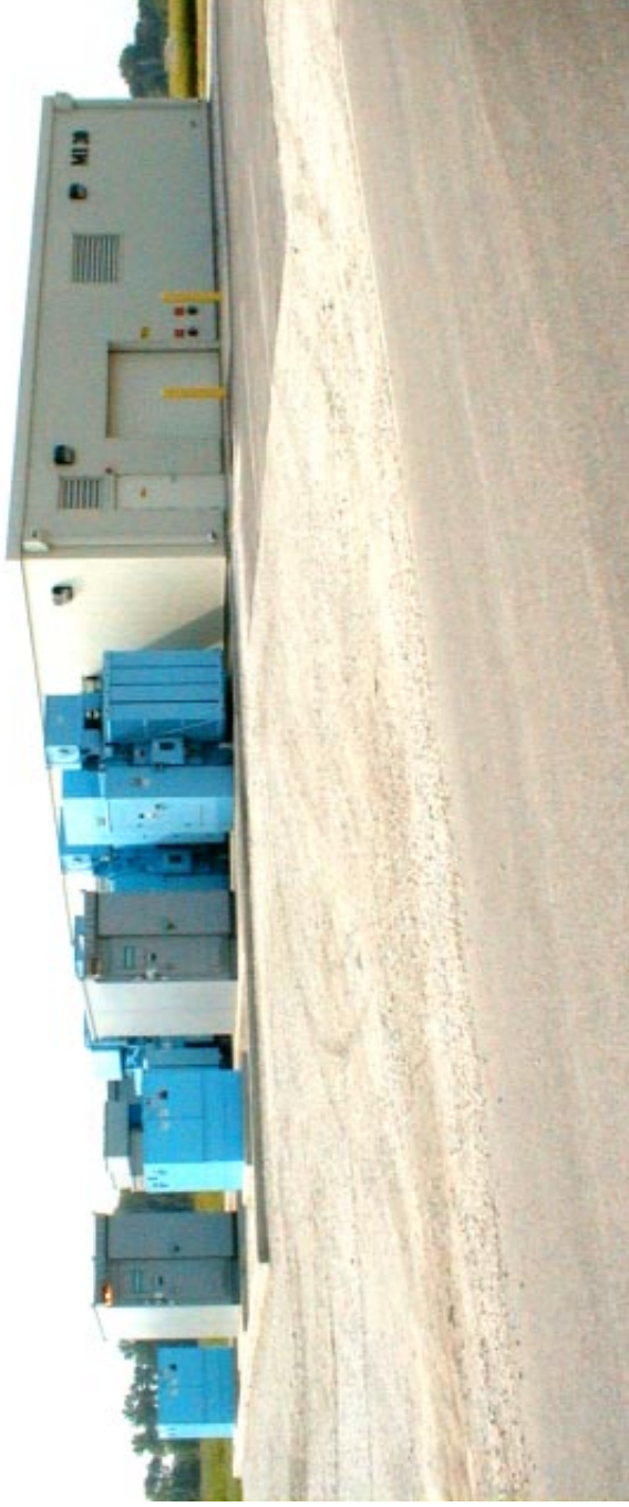
MI-20: One of 6 Fermilab Main Injector Power Supply Buildings
