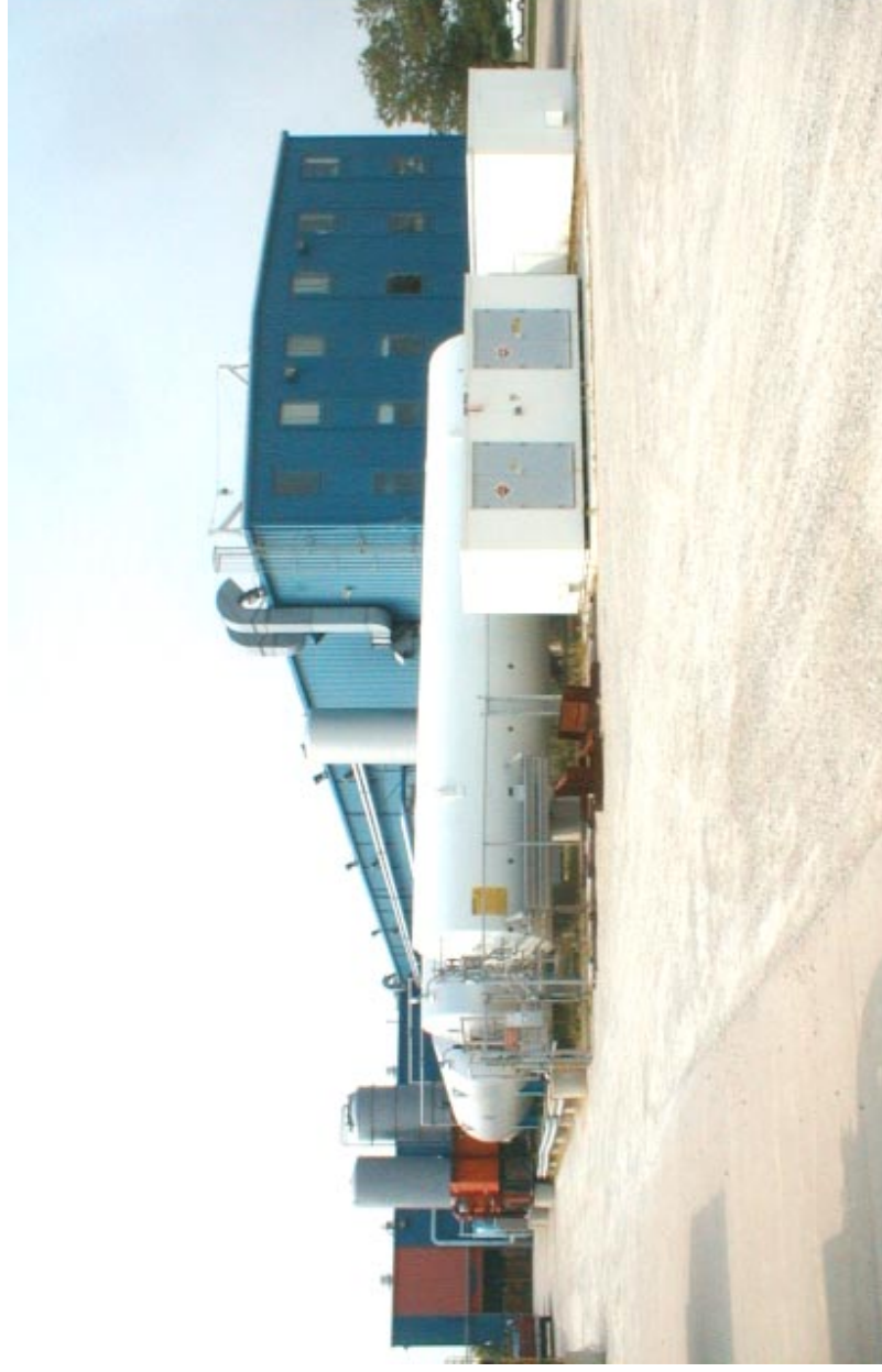
Fermilab's Central Helium Liquefier
